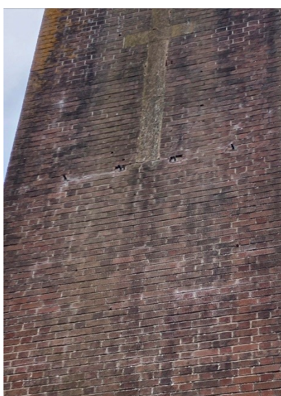
Fig 5 Crack below the west window is long-standing and there is no evidence if it progressing.
