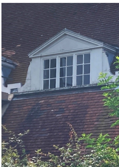
Fig 7 The 'hatch' into the chancel roof space is in need of redecoration and, quite likely, repair.
