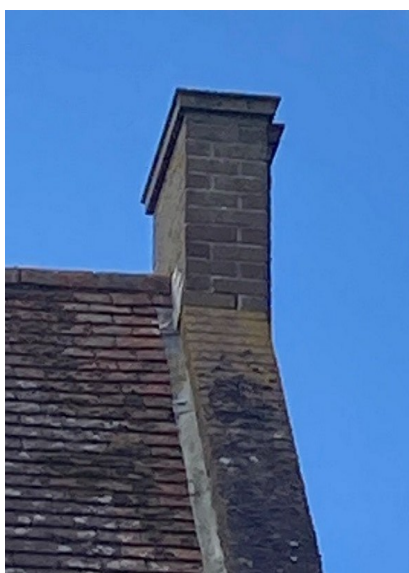
Fig 3 The south east kneeler to the chancel is moving slightly outwards. This is not yet urgent but some 'pinning' is desirable to ensure that the issue does not get worse.
