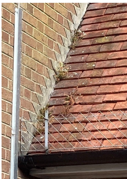
Fig 1 Woody growth in the back gutter to the south dormer.
