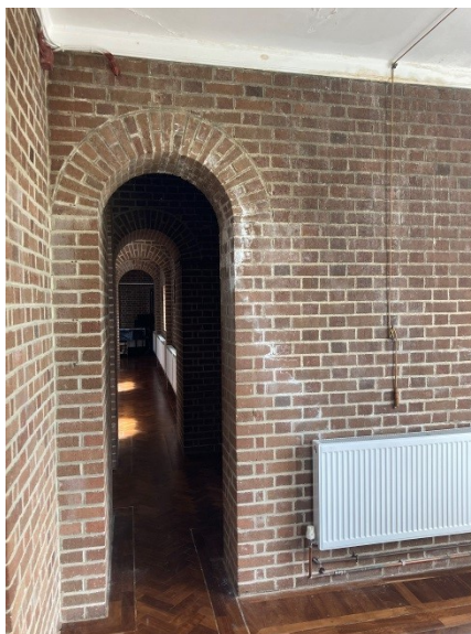
Fig 12 Damp staining at high level in the south arcade below the north wall of the tower.
