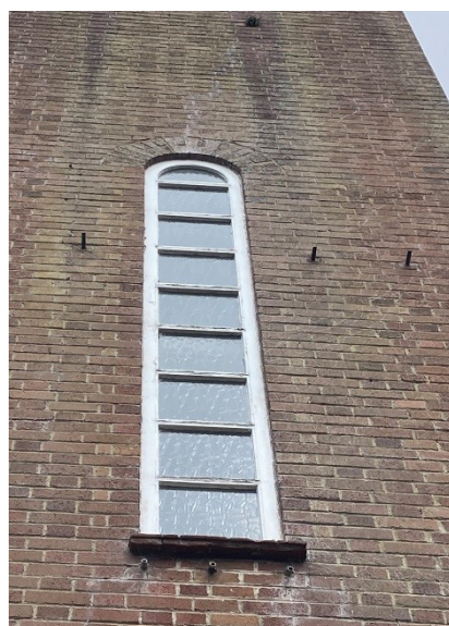
Fig 9 The west window showing need for redecoration. The partial Perspex secondary glazing detracts from the appearance of the window.
